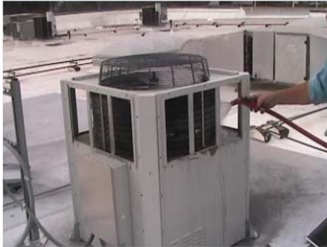
Figure 3. Wash the Heat Exchanger coils
