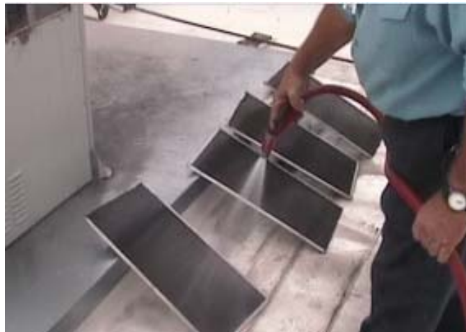
Figure 2. Wash the compressor air filter screens with a water hose
