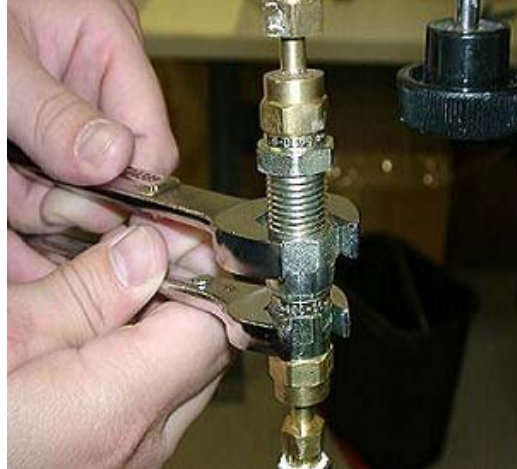
Figure 2. *Note: Using only one wrench to remove this fitting can cause damage to the supply line.
